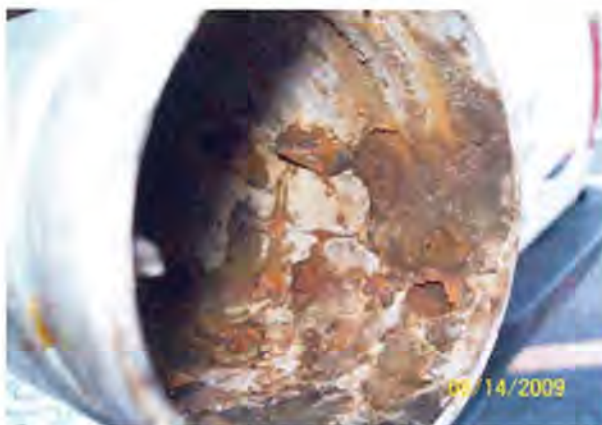
Photo 8: Scale that can form in dry pipe sprinkler systems that can break off and clog pendant-type sprinkler heads. Photo provided by U.S. Automatic Sprinkler Corp.
