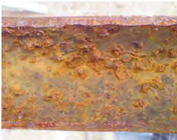
Photo 7: MIC tubercles (biodomes) inside of sprinkler piping. Photo provided by Potter Electric Signal Co.
