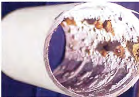
Photo 6: MIC tubercles inside of galvanized Schedule 40 sprinkler piping. Photo provided by Potter Electric Signal Co.
