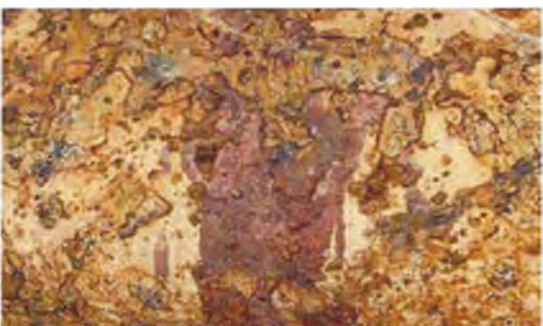
Photo 3: Microbiologically influenced corrosion. Photo provided by Potter Electric Signal Co.
