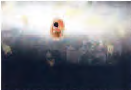
Photo 5: Hole created in sprinkler piping by MIC. Photo provided by Potter Electric Signal Co.
