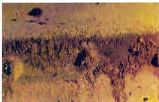
Photo 1: Pitting inside of piping. Photo provided by the American Fire Sprinkler Association
