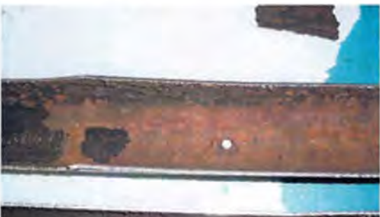
Photo 4: Internal pipe corrosion and hole in galvanized sprinkler piping. Photo provided by Potter Electric Signal Co.
