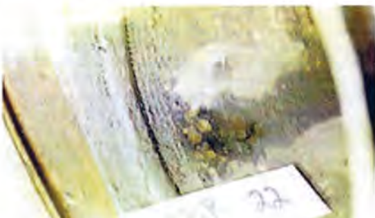
Photo 2: Pitting that remains after chemical cleaning of the pipe to remove tubercles. Photo provided by the American Fire Sprinkler Association.
