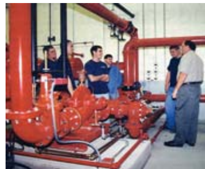
Harold Lawson (right) describes the operation of a fire pump in the TECenter.
