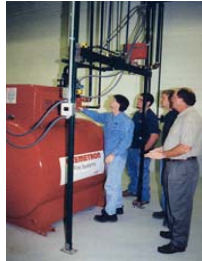
(l to r) Design Technician Larry Dunham, apprentices Matt Coleman and Stephen Gaiser, and Special Hazard Salesperson Harold Lawson take a closer look at a CO2 system in USAutomatic's TECenter.
